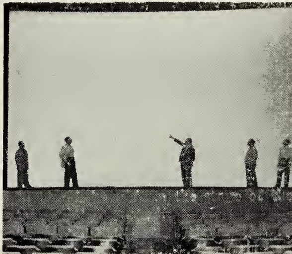
Loew's Poli, Springfield, Mass., was only closed for 36 hours recently while a crew of 40 made alterations and erected the wide screen shown. Seen in front of the screen are Marcell Fasano, production engineer; Joseph Piontek; manager George E. Freeman; John Miller, in charge of rigging the screen, and Albert Fortune, stagehand.
